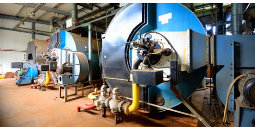
Application examples: Boiler
